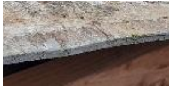
The delaminated ramp edge after 18 month's exposure to weather
